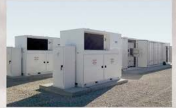
40HC 800KW/524KWH Lithium-Ion Battery
