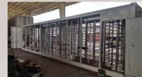
40HC 500KW Lead Acid Battery
